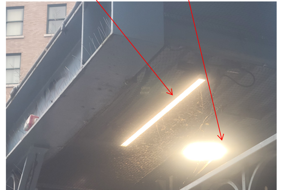
Light fixture at the 3rd Avenue Entrance.
