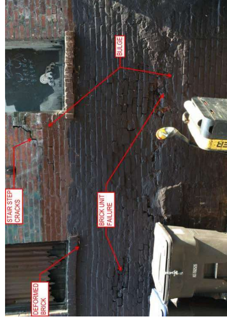
Figure 3: West Wall Localized Failures
