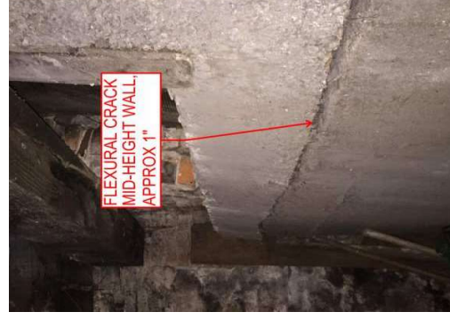
Figure 4: Basement Wall Flexural Failure
