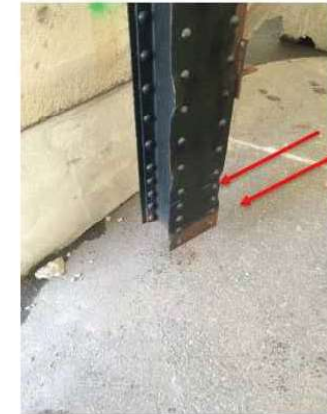
Figure 3. Typ. example of warped Column Base (photo of C B1)
