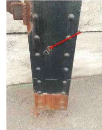
Figure 2. Typ. example of raised rust patches to be repaired (photo of C B2)
