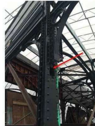
Figure 3. Typ. example of missing corbel (photo of C B8)
