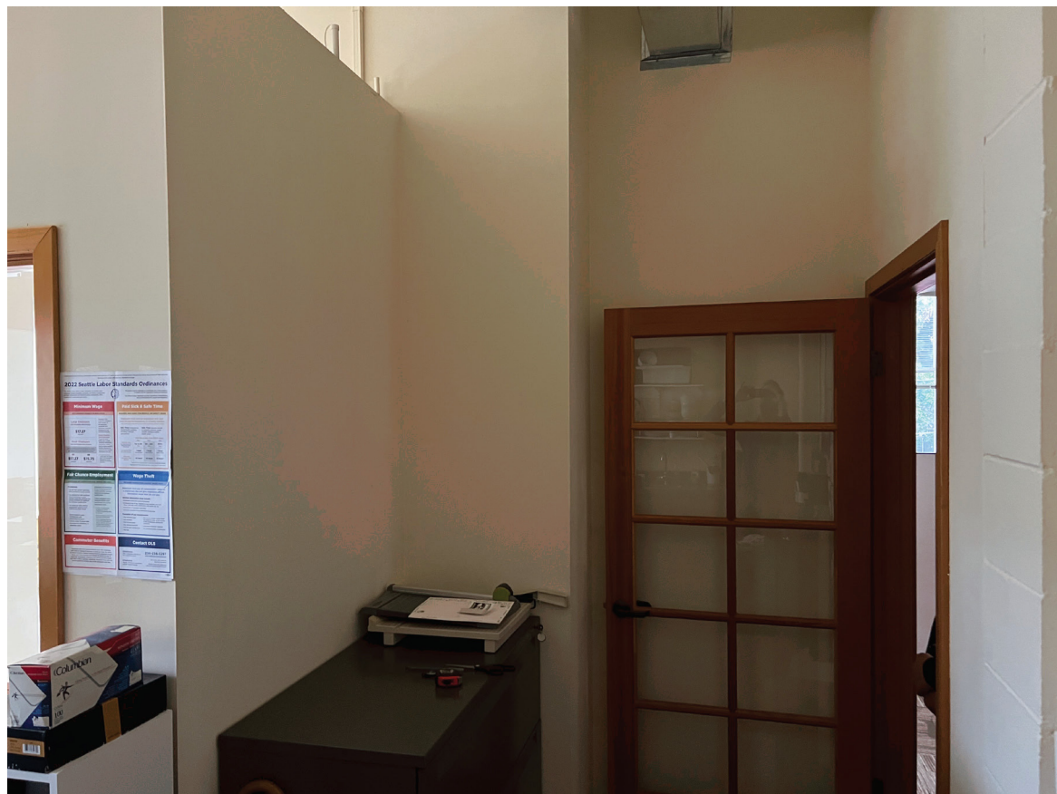
VIEW TOWARDS NORTHEAST. PARTITION WALL AND DOOR AT RIGHT TO BE REMOVED.
