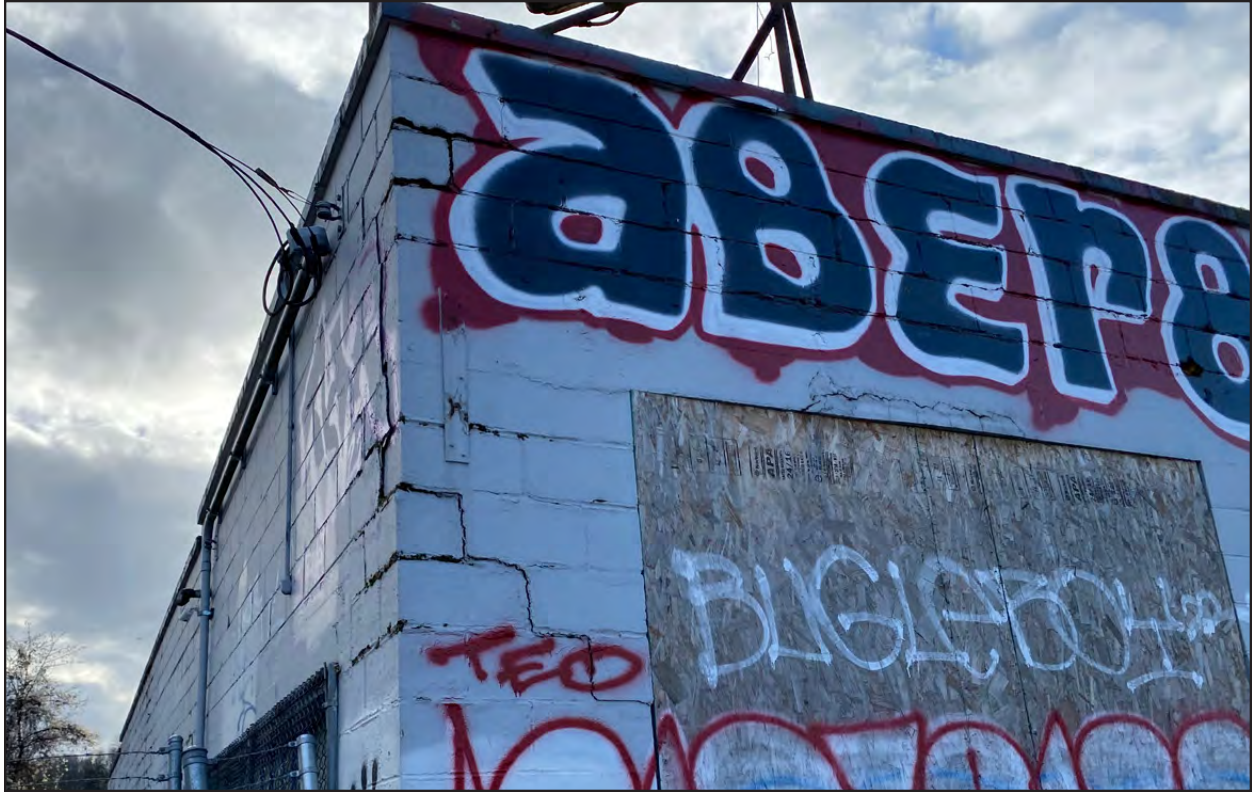
Figure 22 • 1265 S King Street, condition of CMU
