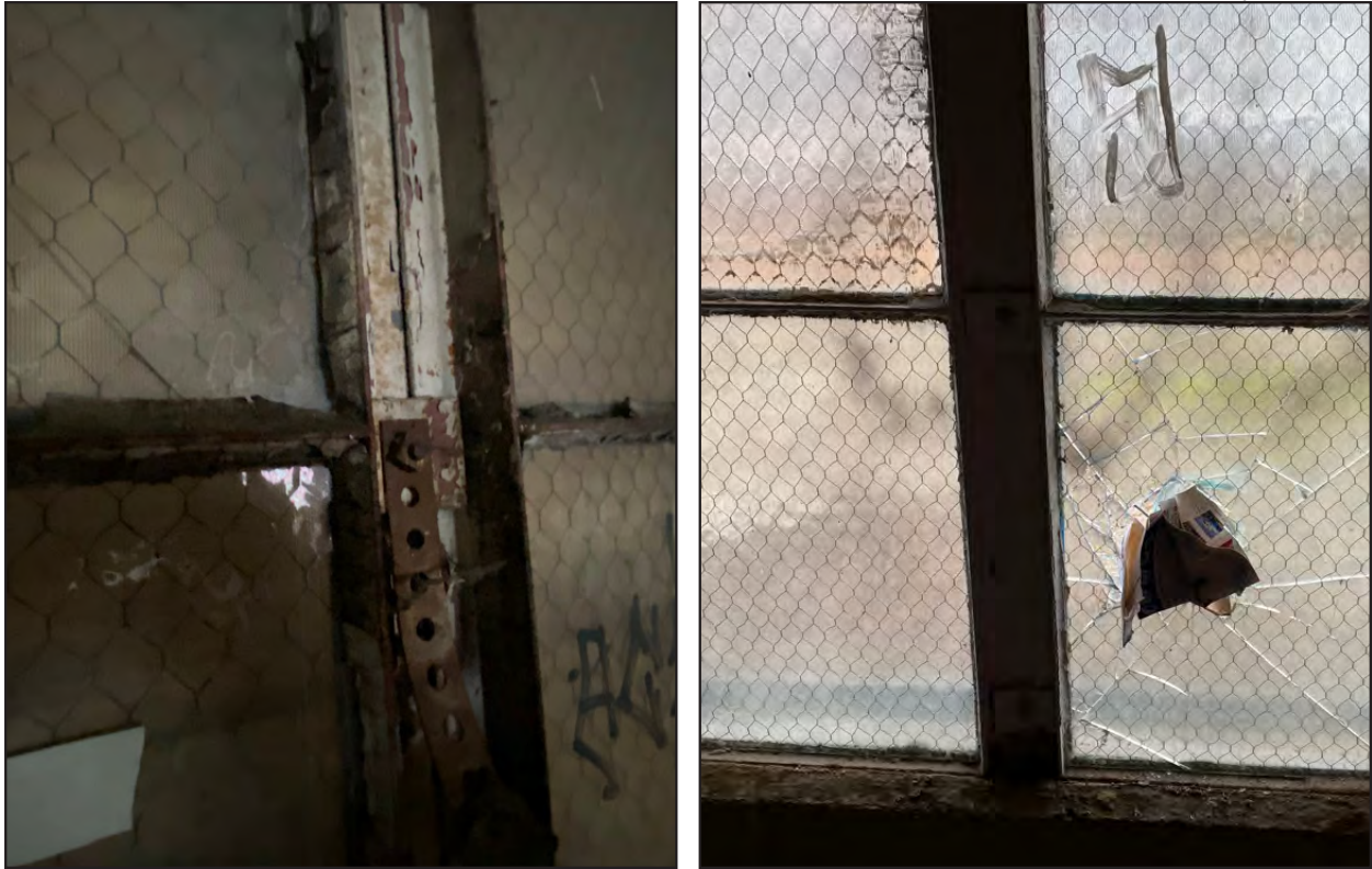
Figure 24 • 1265 S King Street, condition of windows
