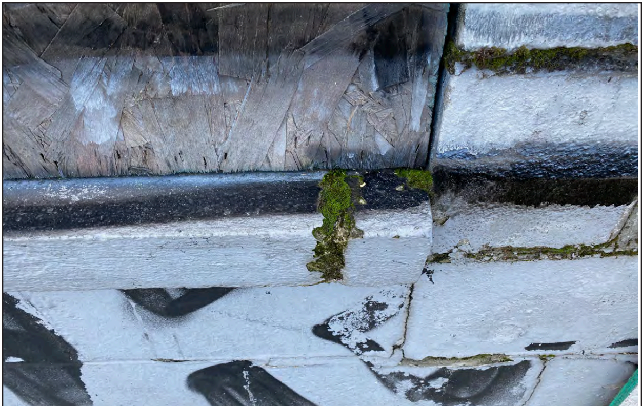
Figure 25 • 1265 S King Street, condition of windowsill
