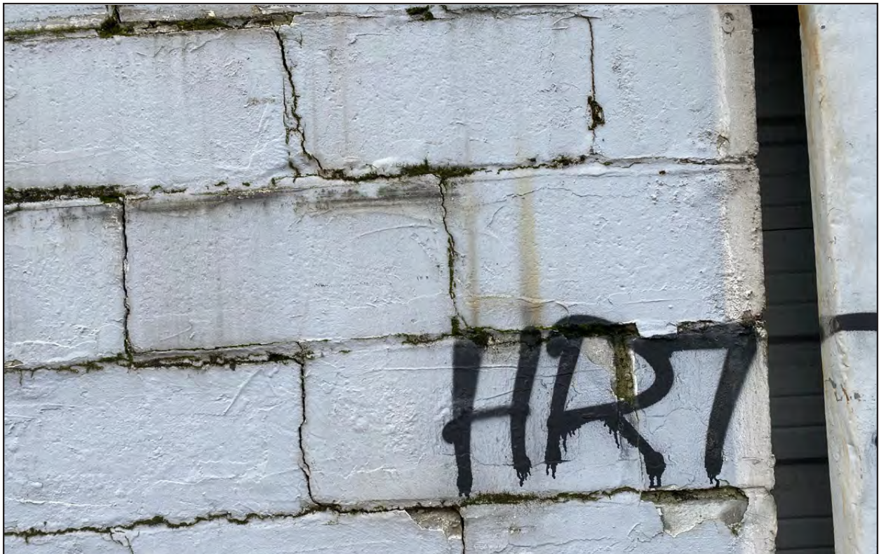
Figure 23 • 1265 S King Street, condition of CMU
