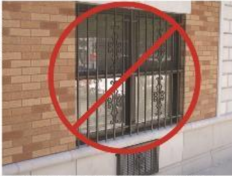
Prohibited bars installed on the building facade
