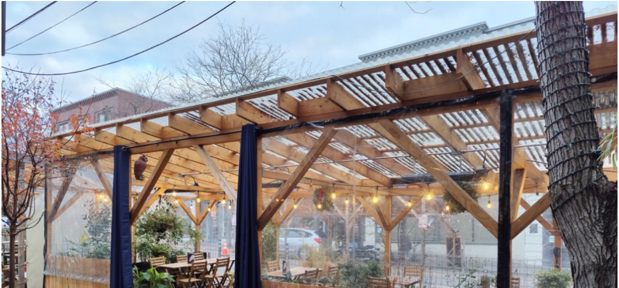
Photo 11: We will be replacing our existing plastic sheeting on our structure. This photo shows how the roof is currently constructed.
