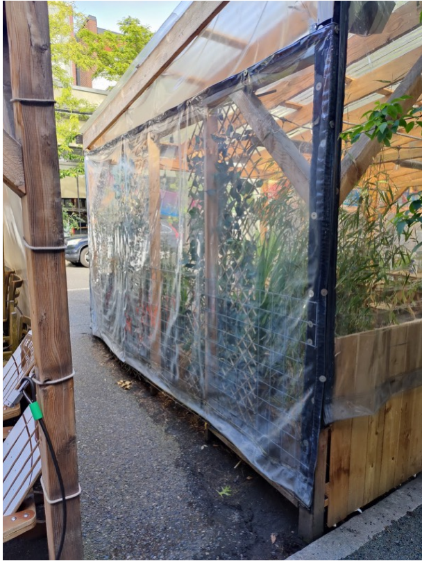
Photo 19: The photo to the left shows the existing metal fencing covered by the rollable rain flaps.
