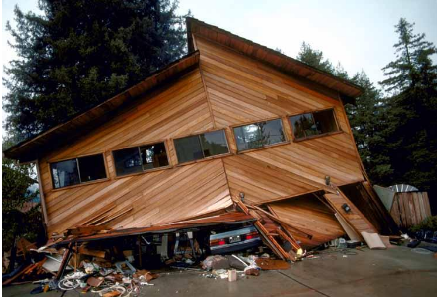
Figure 28. Home Damage Due to Soft Story
