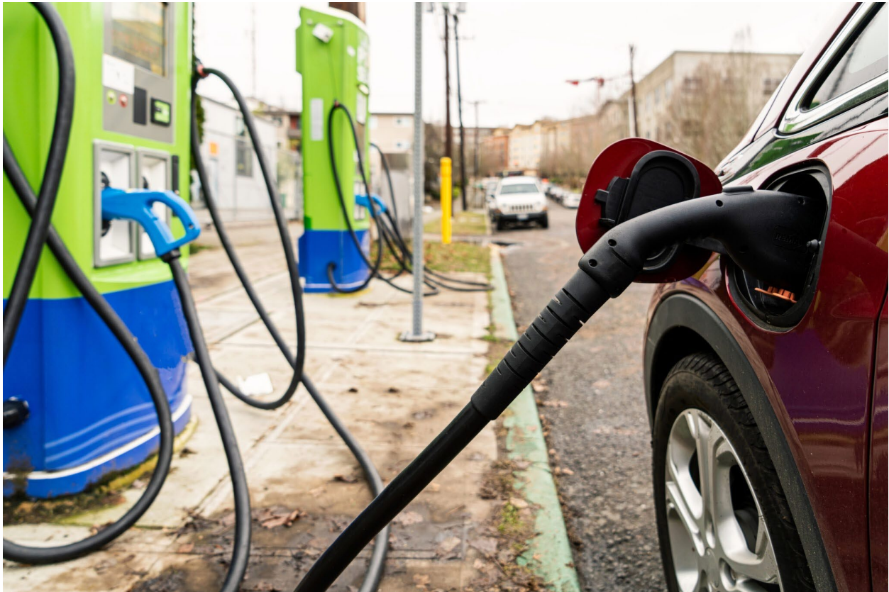
Expanded City Light EV charging stations are available across Seattle.
