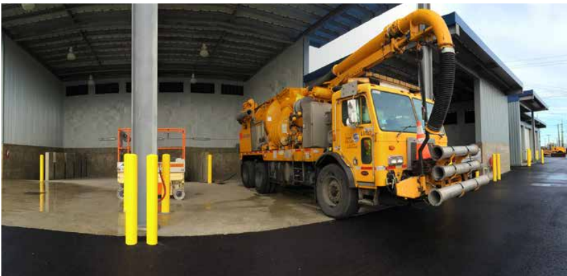
South Service Center treatment facility
