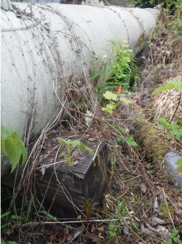
Figure 12. Potentially contaminated wood saddle underneath the penstock that will need to be replaced if penstock is left in place.
