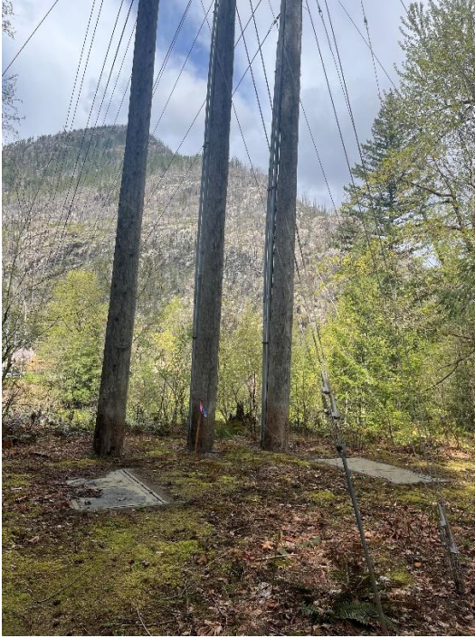
Figure 1. Power poles, transmission lines, and underground transmission line vaults adjacent to the Skagit River.
