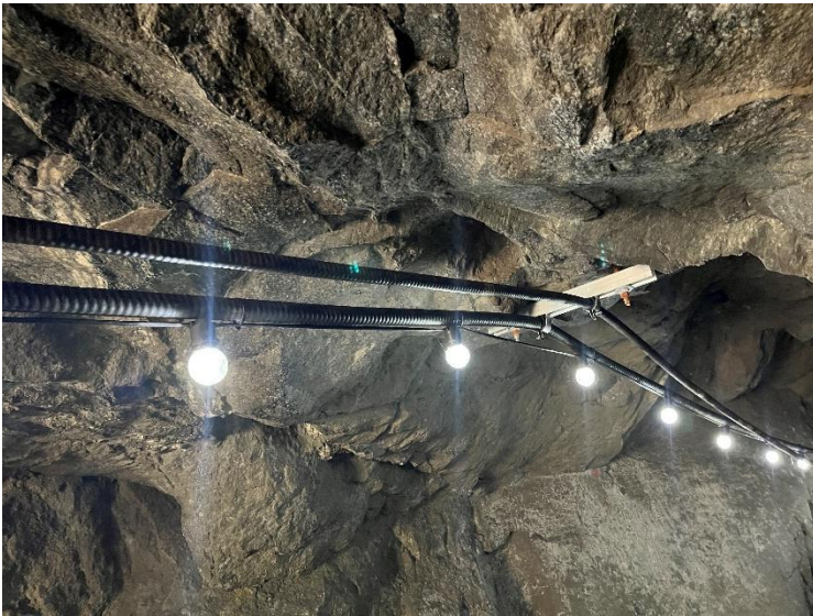
Figure 7. Electrical conduit, lights, telephone line, and anchors in the penstock tunnel.
