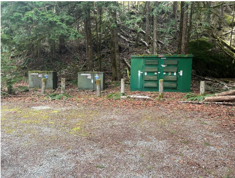
Figure 2. Transformers and cement bollards adjacent to the Newhalem Powerhouse.
