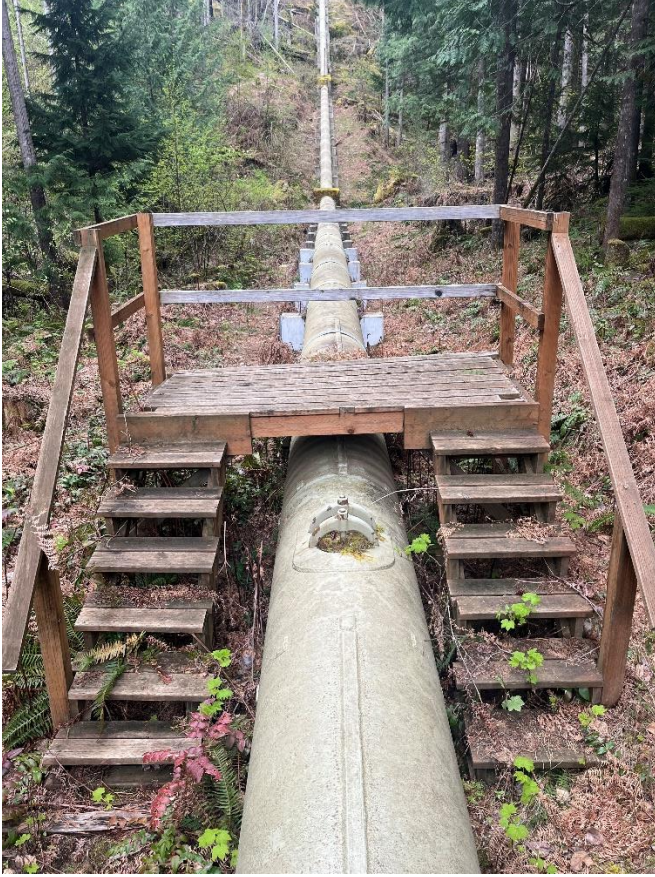
Figure 4. Viewing platform constructed of treated lumber on the lower portion of the penstock.
