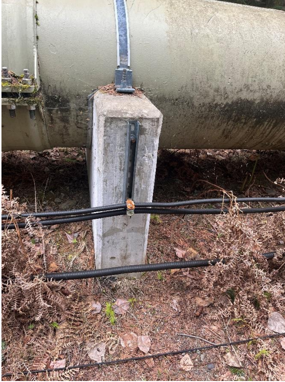
Figure 3. Electrical cables and conduit attached to penstock saddles and telephone line laying on the ground adjacent to the penstock.
