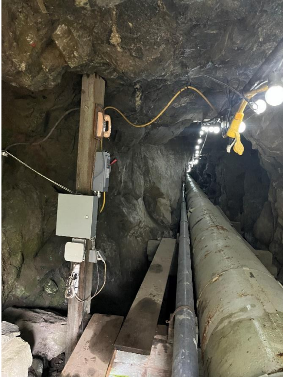
Figure 6. Telephone, circuit breaker, lights, and six-inch PVC pipe inside of the penstock tunnel. The elevated planks providing access and a small portion of the wood cradles are also visible.
