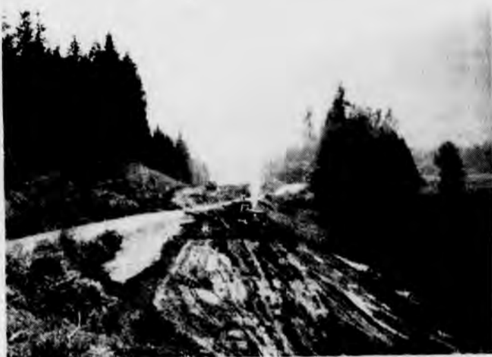
WORK RESUMED ON BAKER ROAD The county project on the Baker Lake road above the Burpee Flat, is now in full swing again with heavy equipment moving earth to re-align and grade the old roller-coaster right-of-way. It is just part of the improvements scheduled for this highway.
