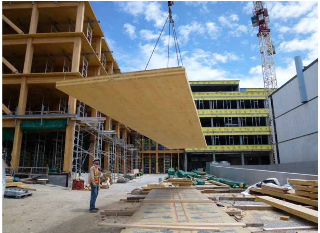
Cross Laminated Timber project at the University of British Columbia, Canada. Source: Structurlam
