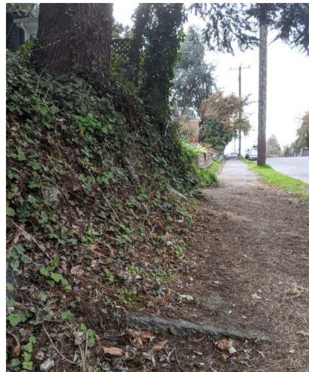
Tree roots encroach into existing sidewalk, significantly lifting the sidewalk and compromising accessibility to the adjacent residential neighborhood.
