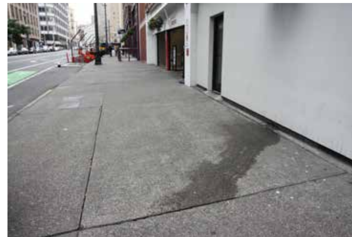
In this case, may only be overhead plant irrigation spillage.
