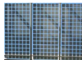
PV panels on roof deck
