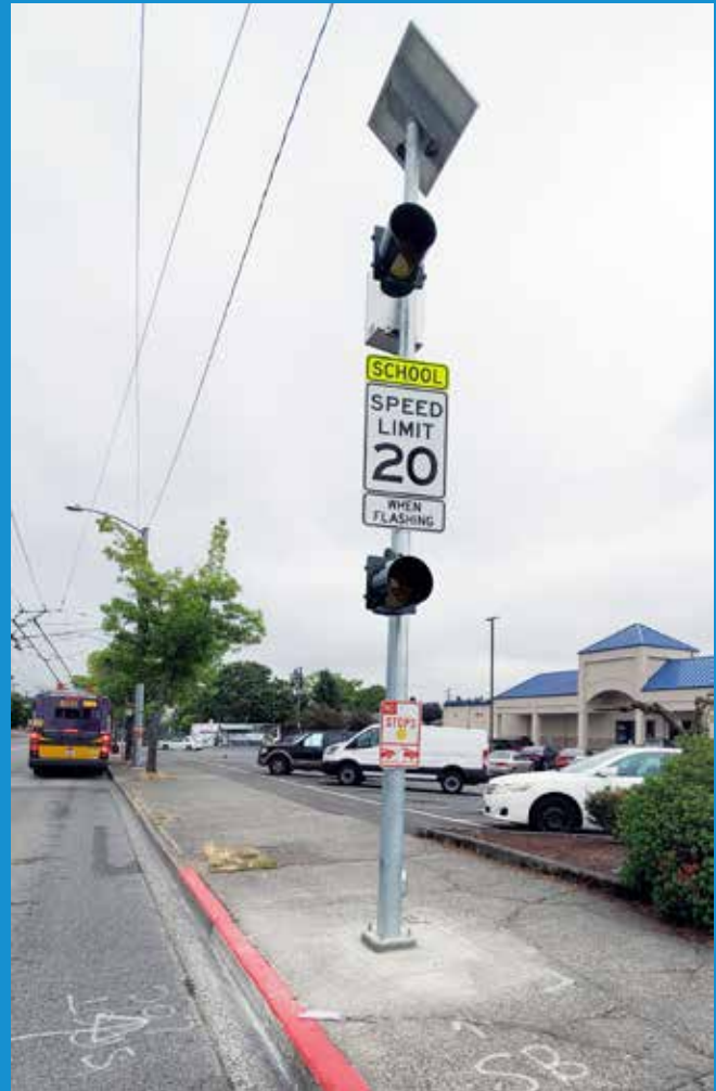
20mph flashing beacon on S Henderson St
