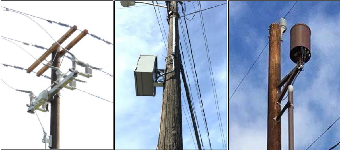
Figure 2: Pictures of a pole-mounted switch, a communications enclosure, and a small wireless facility (left to right)
