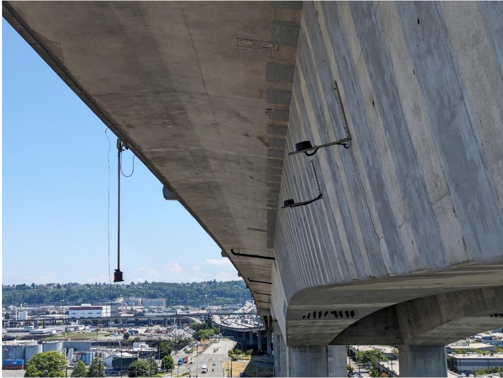
Figure 6 - View from UBIT of the exterior of the bridge, showing strips of CFRP strengthening
