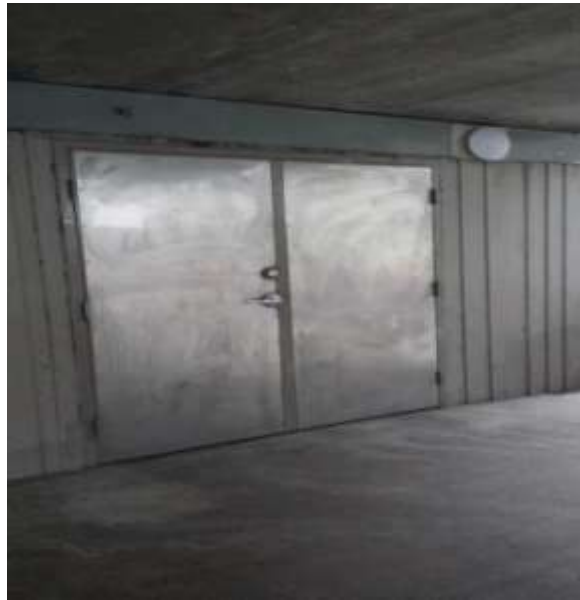
These recently installed doors for the storage area below the underpass are graffiti resistant.
