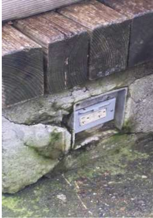
Broken and exposed outlet socket that has been reported (work order completed) by park rangers several weeks prior.
