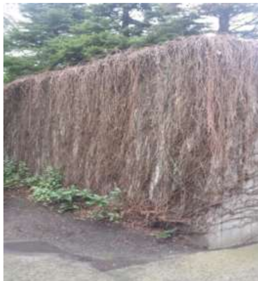
Overgrown vines (not maintained) cover many concrete structures.
