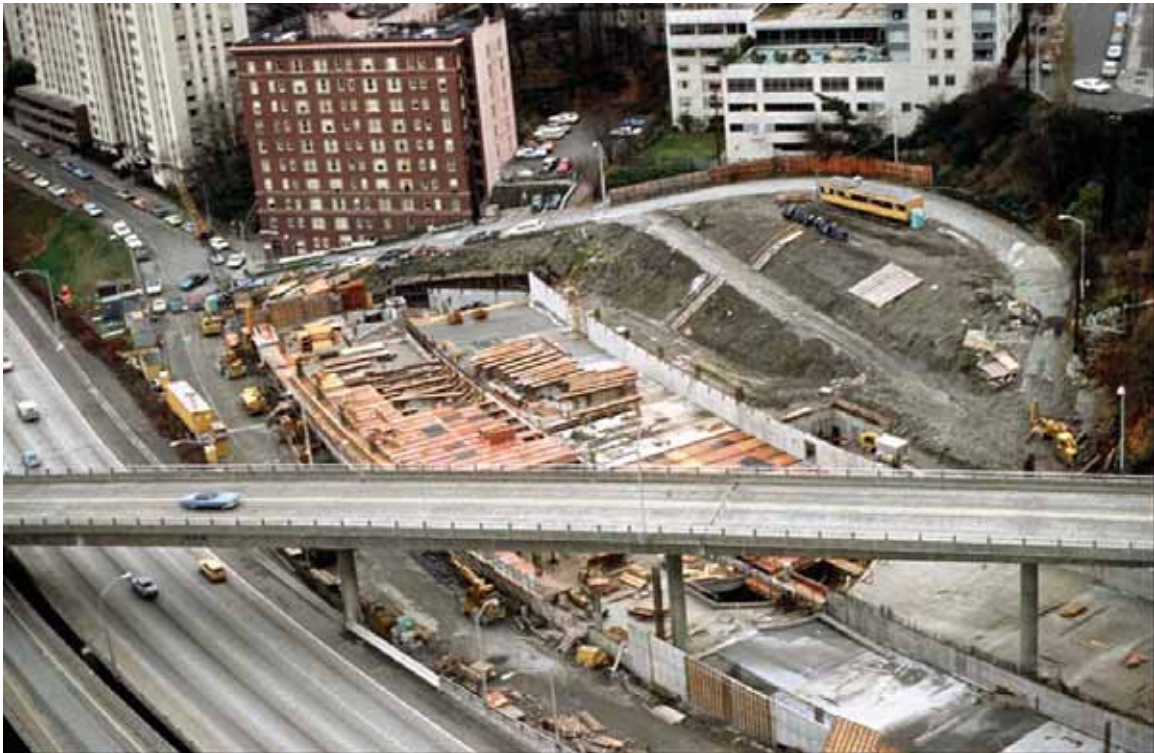
Fig. 115. View northeast of East Plaza construction site, Freeway Park, ca. 1975. (College of Architecture and Urban Planning Visual Resources Collection, image 06617w00.)
