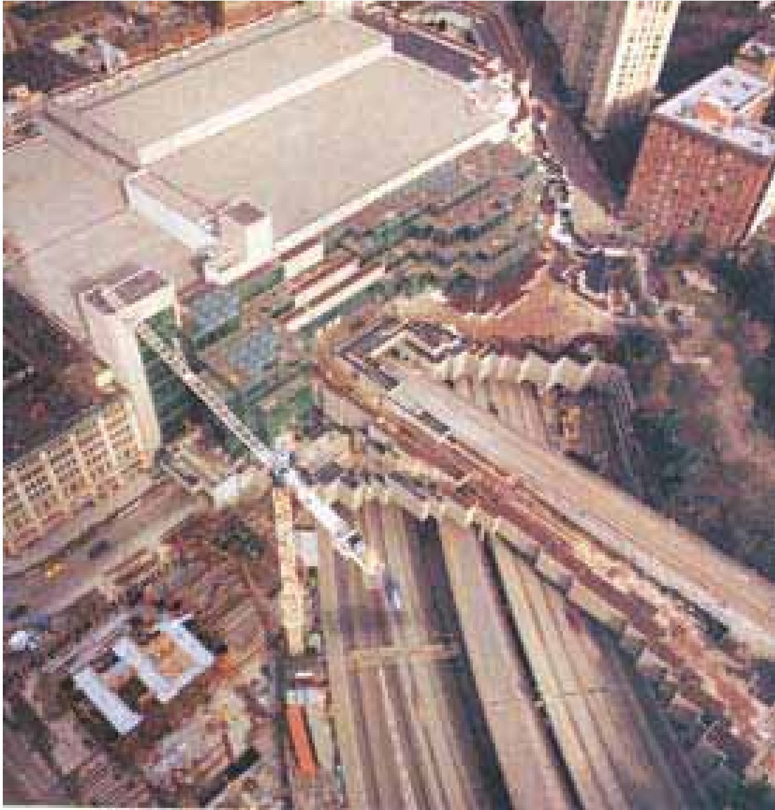
Fig. 100. Aerial view of the construction of the Washington State Convention Center, view looking north with East Plaza to the east, Washington State Convention Center and Freeway Park, 1989. (Bordenaro 43.)
