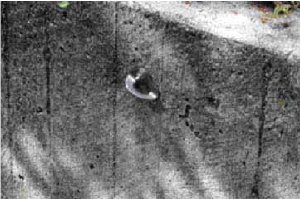
Fig. 61. Typical example of a wall anchor installed in board-formed concrete wall, Freeway Park, 2003. (Photo by authors.)
