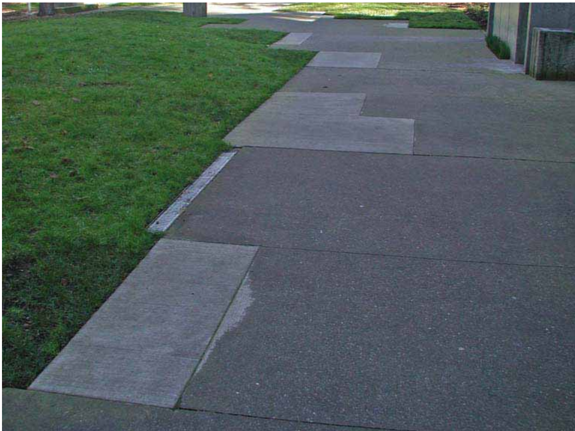
Fig. 85. East Plaza paths showing mismatched concrete pours, view north from south side of restrooms, Freeway Park, 2005. (Photo by authors.)
